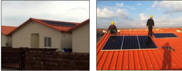
Fig.28: (Example 3) Korean Village, Erbil. The color of PV is not matched with the roof colour. (Source: Researcher)
